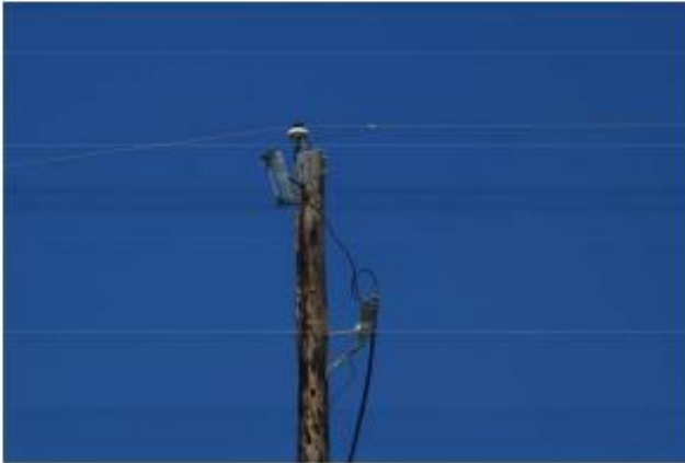
Single Phase Riser
