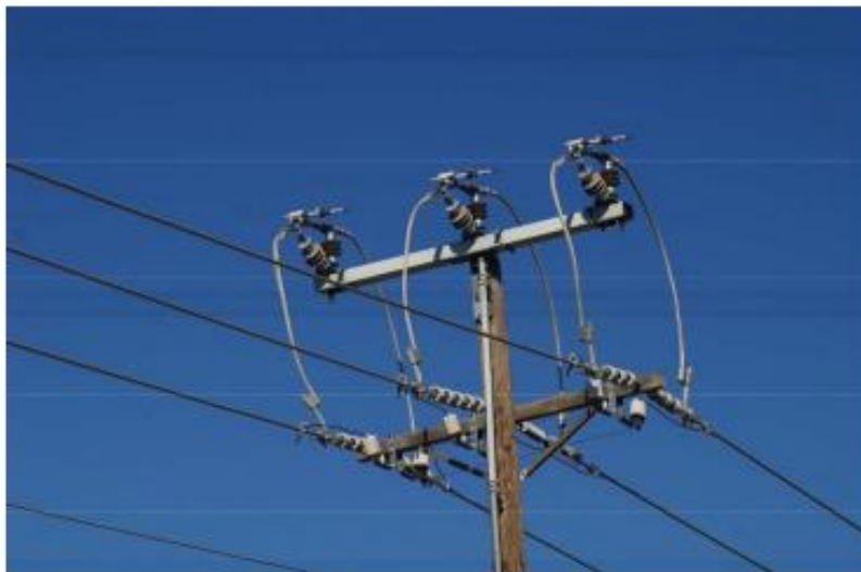
Air Break Switch
