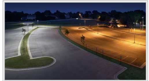
Installation of LED parking lot lights (left) compared with HPS lights (right) shows the difference in color appearance and distribution.
