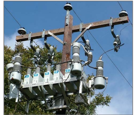
Pictured: Capacitor Bank
