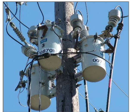
Pictured: Transformer Bank
