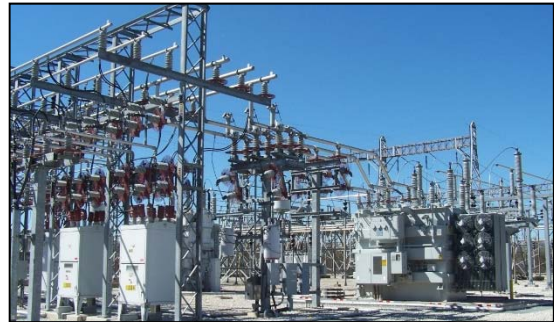
Pictured: Substation equipment
